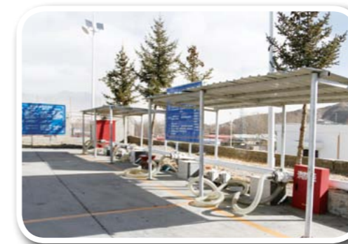
Sun roof for oil unloading platform
